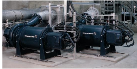
Figure 2. Grundfos dry-pit submersible sewage pumps.
