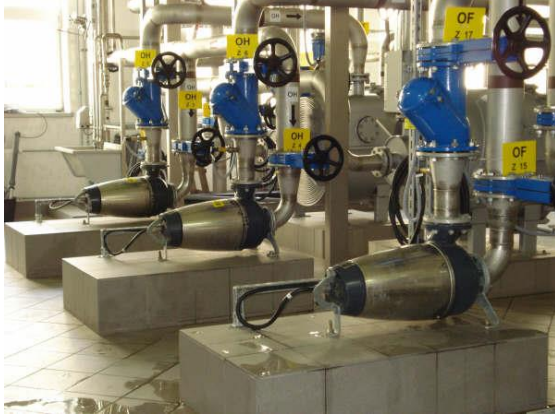
Figure 10. Grundfos sewage pumps horizontal mounted on pre-cast foundations
