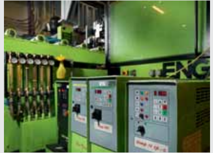
Typical thermic unit for cooling
