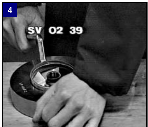
Remove worn wear ring by loosening all way round (to protect impeller neck).
